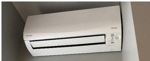
New office heater
